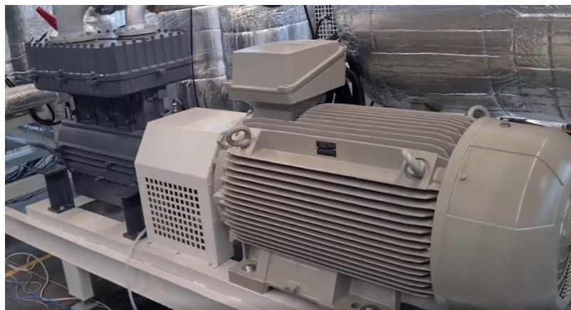
Figure 3 — Compressor and motor arrangement.
